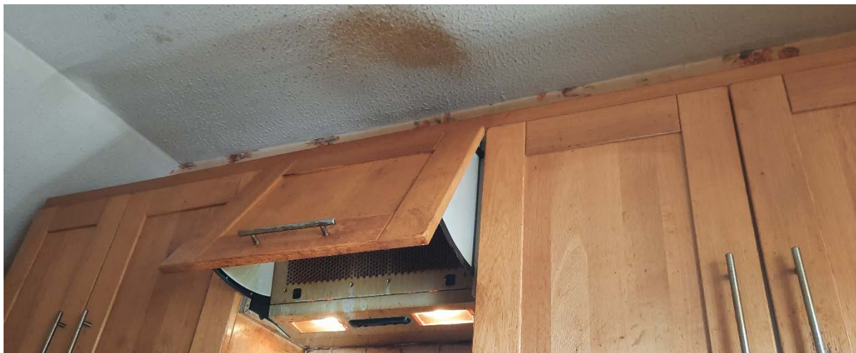
Figure 5 - Damp and mould growth from an extractor fan without a duct to outside.
