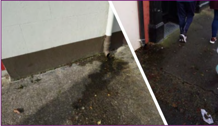
Figure 5 Photos highlighting an example of downpipe discharge onto the public footpath causing additional problems for older people and people with mobility issues. (Toler Street)
