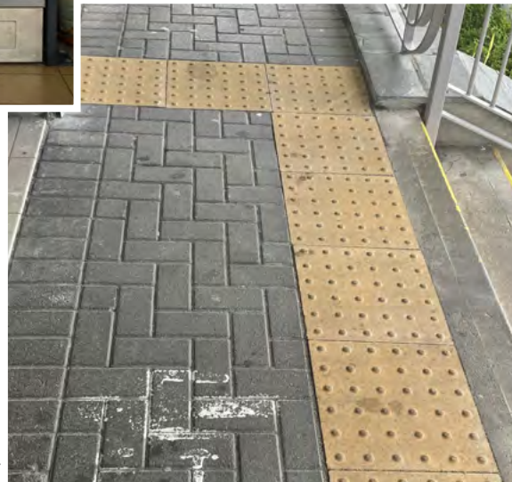
► Tactile Pavement for customers to identify steps.
